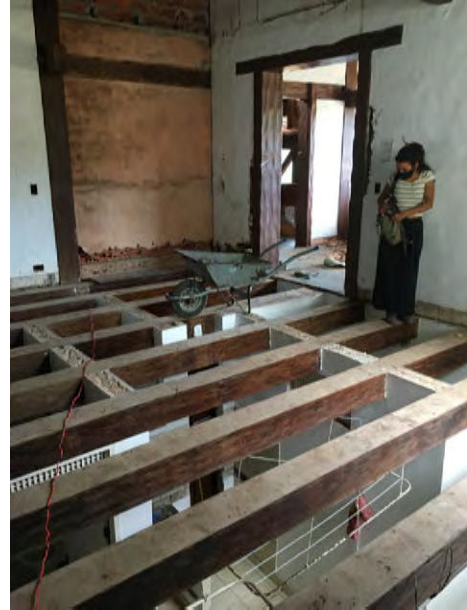
Natalia Lessa on site during deconstruction. The team spends roughly 30 days per house in which they take inventory, assess quality, deconstruct and sell materials on site.
