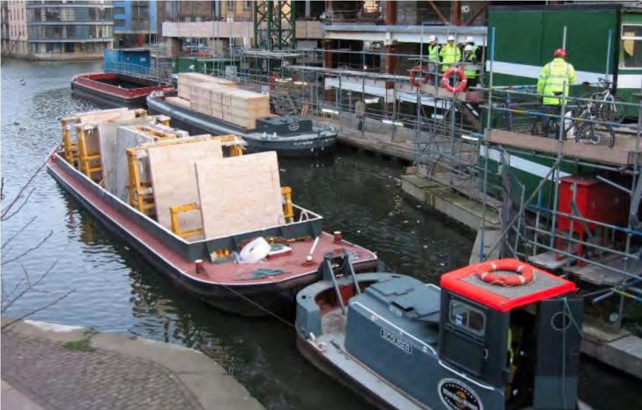
Development in King's Place, London N1: At a congested urban development site, barges delivered material to be stored on-site without taking up room. (CLIG AtoH Ltd. Construction Logistics Improvement Group, Meeting 9)
