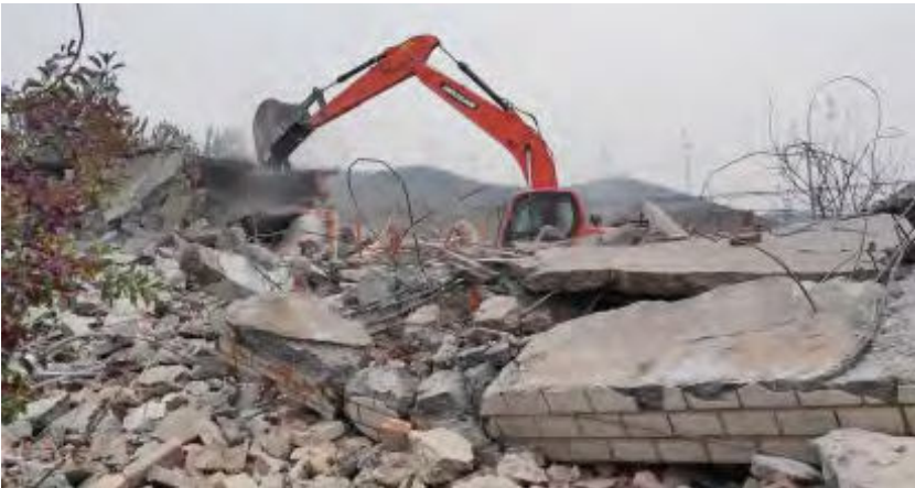
Reinforced concrete and brick houses are considered unreclaimable, so they are demolished and destroyed completely.
